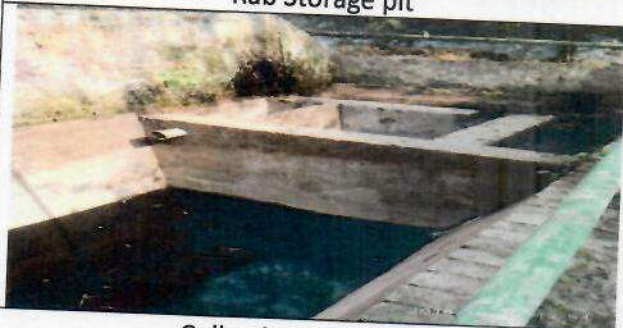
Collection tank of ETP
