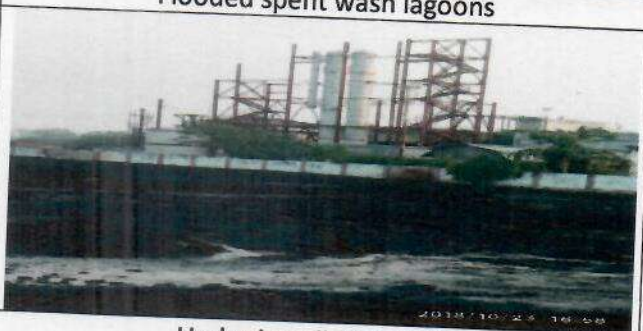
Under installation MEE
