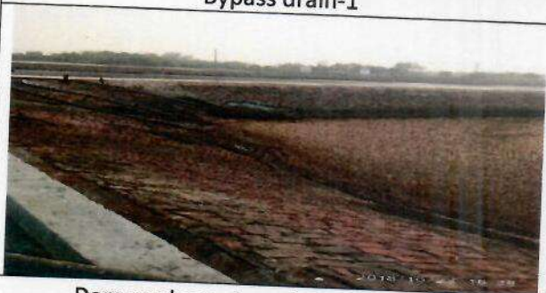
Damaged spent wash storage lagoon
